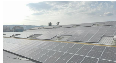
Rooftop Solar Panel
