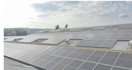
Rooftop Solar Panel
